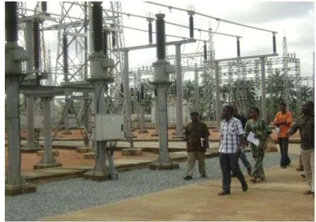
Picture 15: Umuahia 2x30/40MVA- 132/33 KV Substation Abia
