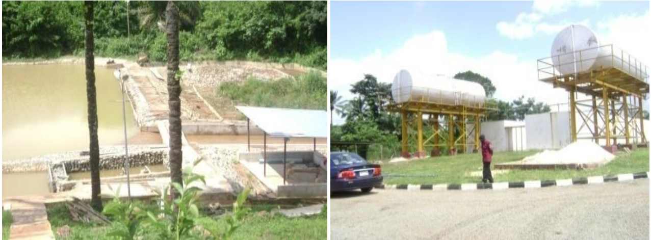
Picture 14: On-going Construction of Water Project at University of Nigeria Teaching Hospital, Enugu
