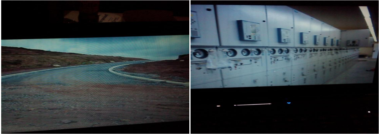
Picture 1: On-going Road Works & 33/11 KVA Electrical Power Supply at Guzape District Lot II
