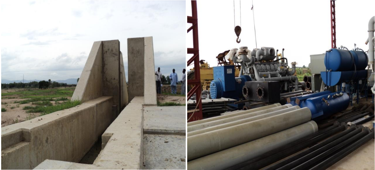
Picture 12: Chouchi Diversion Dykes & Electrical Equipment on site for the Irrigation Project
