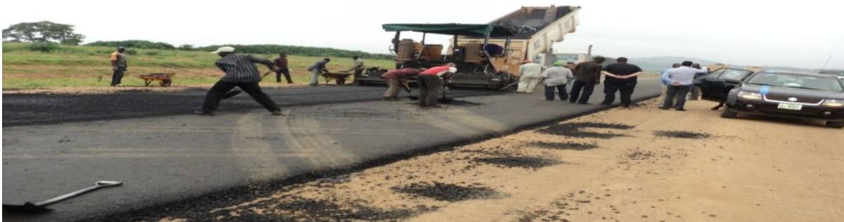
Picture 4.7: Ongoing construction work of the dualization of Ibadan – Ilorin Road (Route A2) Section II: Oyo – Ogbomosho Road
