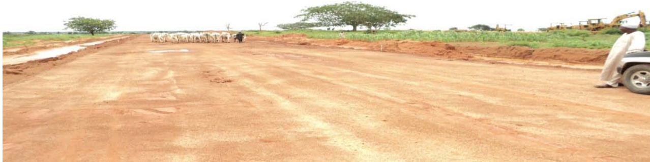
Picture 4.9(b): Construction of Embankment in progress in Sector 6 of the project
