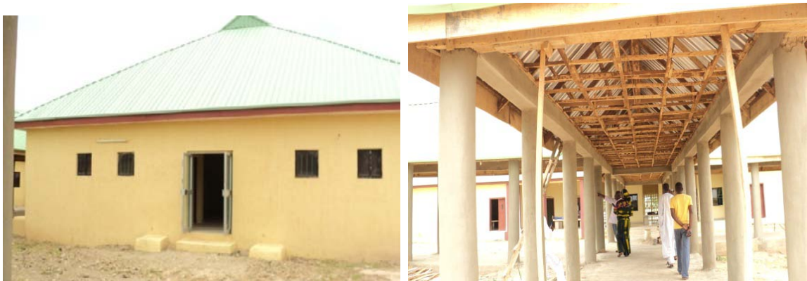
Picture 4.25: Construction of Ward and Walkways at the Argungu Health Centre, UDFUTH, Sokoto
