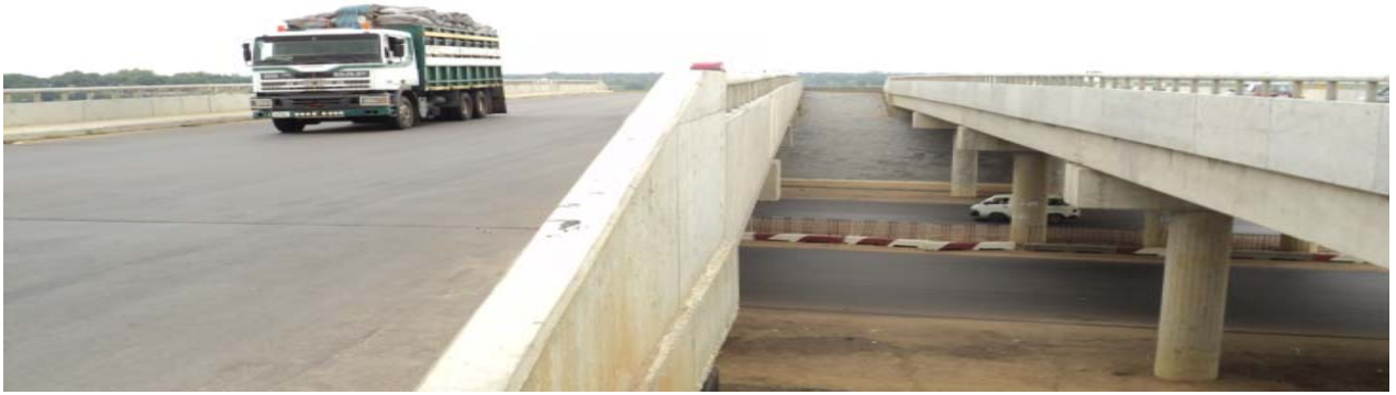
Picture 4.5(a): The flyover bridge at the Kano Western Bye-Pass, almost completed
