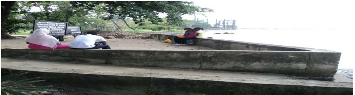
Picture 4.39: Completed Land Reclamation and Structure Protection Works at the University of Lagos
