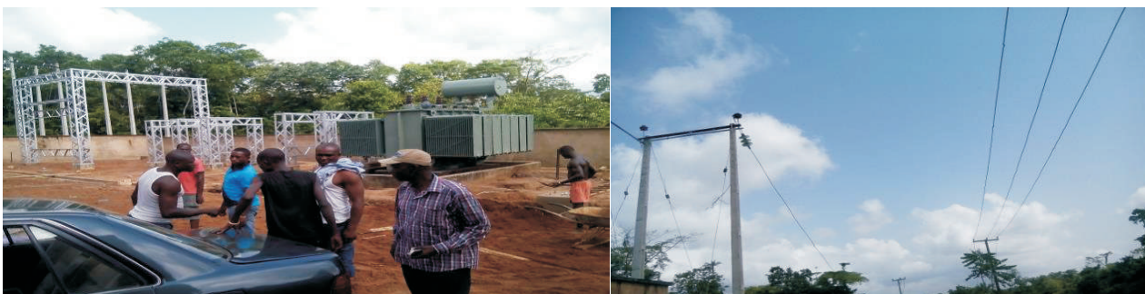
Picture 18: The Gantry work and installed Transformer, Poles and Strings
