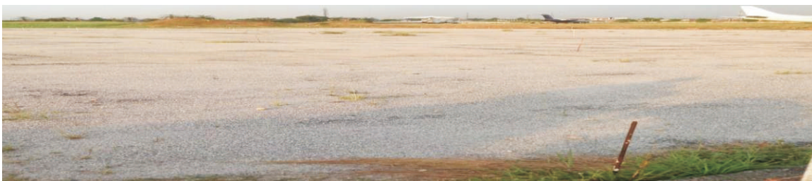
Picture 7: Ongoing rehabilitate and upgrading work at General Aviation Terminal Apron for parking aircrafts at Lagos Airport
