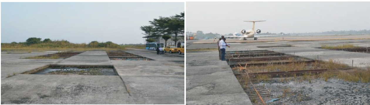
Picture 3: Construction of partitions and parts of slabs laid at the Apron expansion site of the Airport
