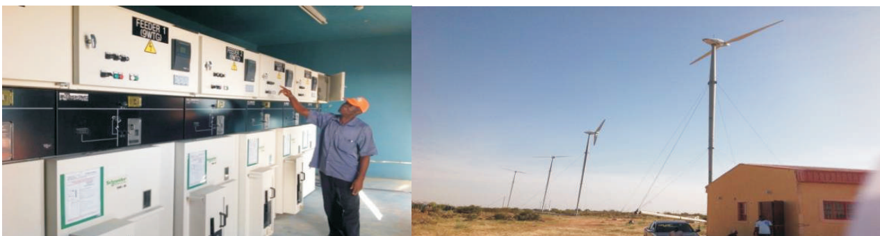
Picture 15: The Installed Medium Voltage Equipment and Commissioned Turbines at Katsina Wind Farm
