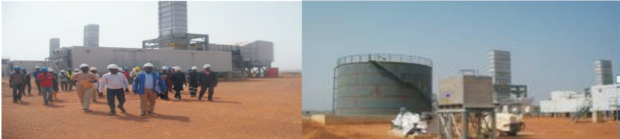
Picture 28: Fully installed turbine and tank at the power station, Kaduna
