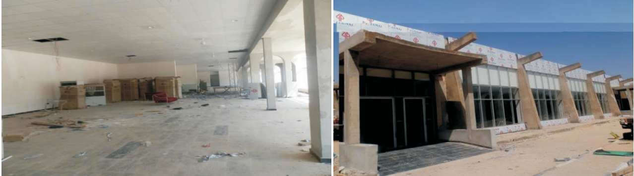
Picture 4: The on-going renovation, upgrading and refurbishment of Maiduguri Airport Terminal Building
