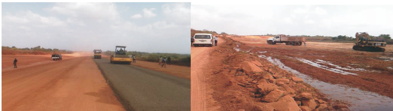
Picture 12: On-going Road Construction Work at Ibadan - Ilorin Dual-Carriage Way: Section II
