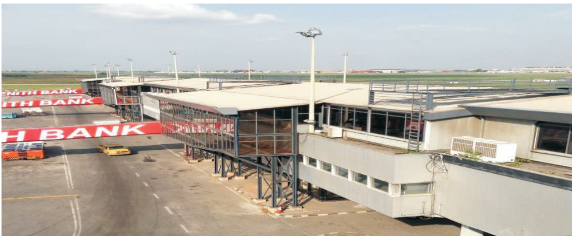
Picture 6: Ongoing Expansion and Upgrading of MM1A Terminal Building at Lagos Airport
