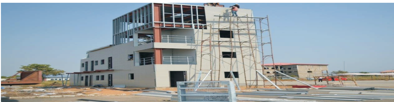
Picture 27: Ongoing Construction of Fire House at Fire Service Academy, Sheda– Abuja
