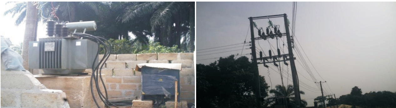
Picture 33: Some of the procured/installed transformer and electrification project at AmapuNtigha and Ovungwu communities of IsalaNgwa LGAs
