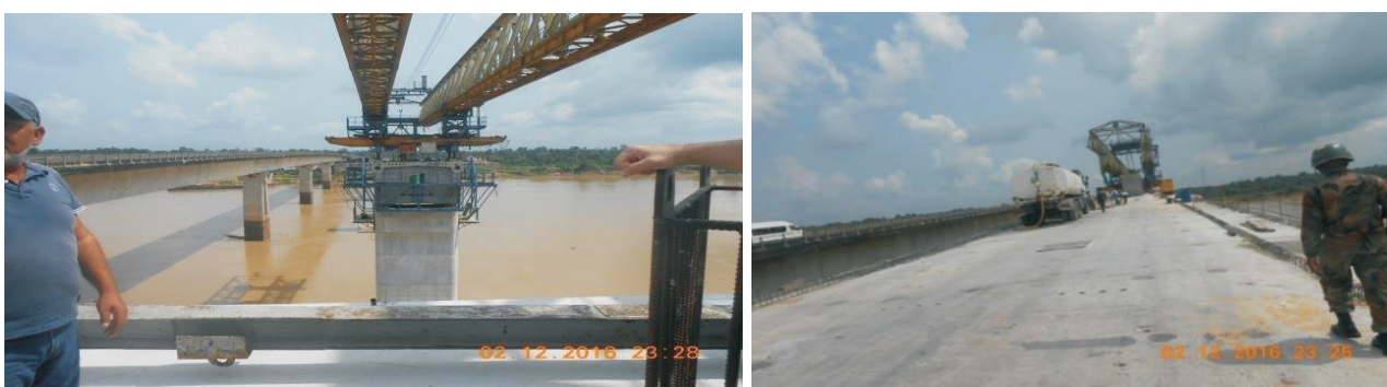
Picture 36: Ongoing works on Kaiama Bridge of the East West Road Section II Sub-Section II
