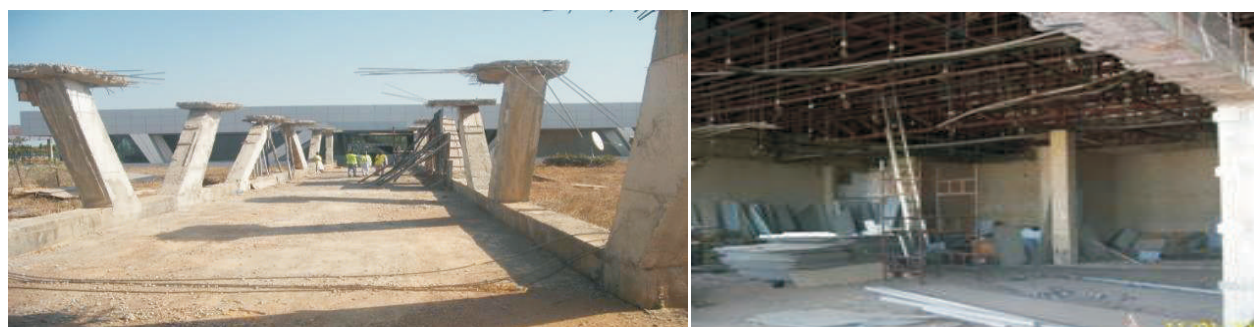
Picture 8: Abandoned Terminal Building at Kaduna Airport
