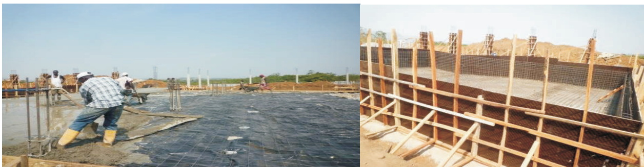
Picture 34: Ongoing Construction work of Sporting Facilities Complex at the Military Pension Board, Abuja
