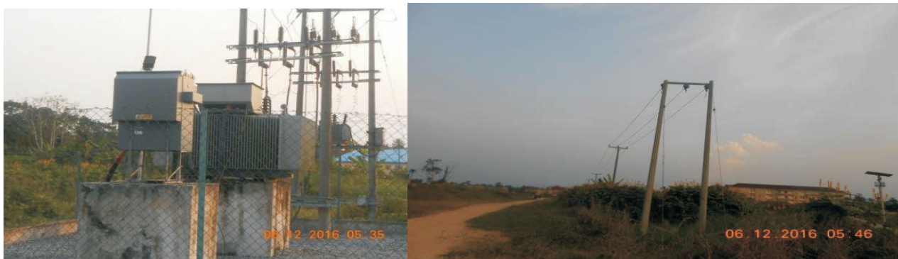
Picture 17: Construction of 33KV Transmission Line and Installation of 2x2.5 MVA, 33/11KV Substation at Federal University, Otuoke
