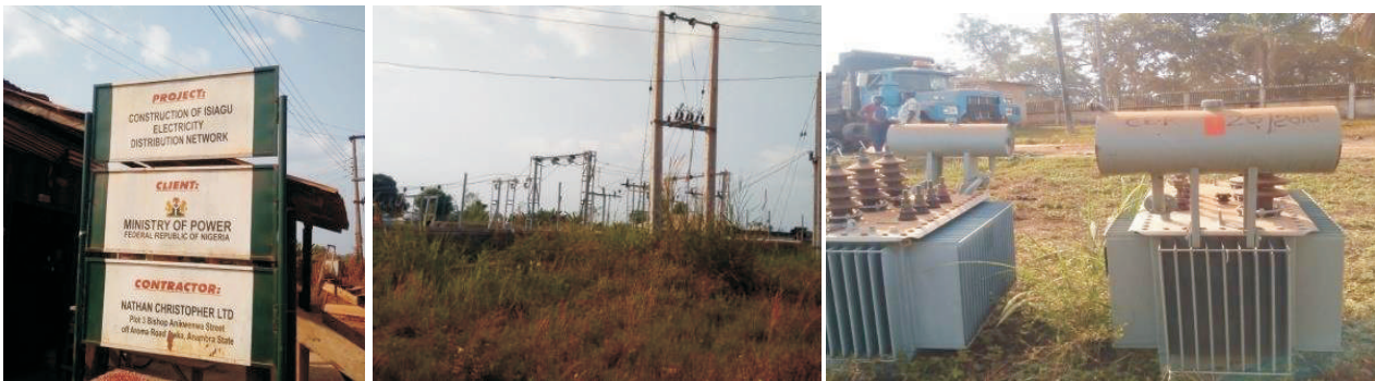
Picture 16: Completed Ishiagu Substation & stolen transformers at the Police station
