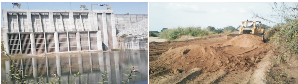
Picture 38: The Completed Right Embankment with the Intake Structures and the On-going clearance of the Access Road to the New Resettlement Birama Community
