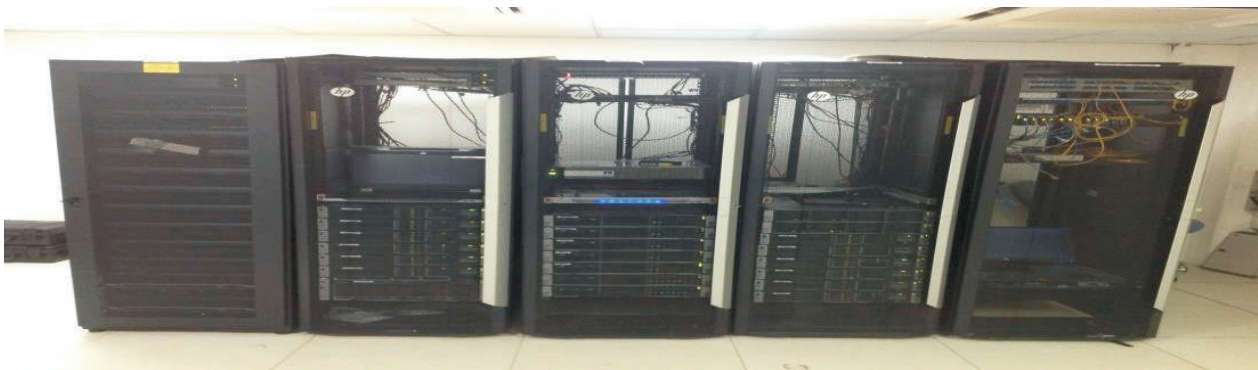
Picture 31: The Intelligence Data Centre platform installed the at Police Headquarters, Abuja
