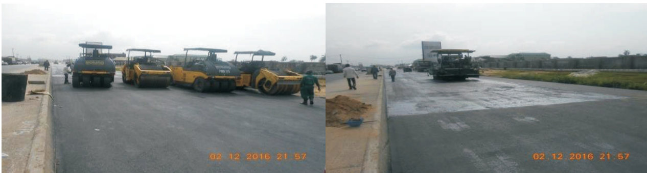
Picture 35: Ongoing wearing course at East West Road Section I, Sub-Section II
