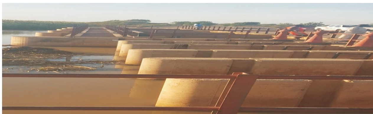
Picture 36: Serviced radial off take/ scour gates at Hadejia Barrage, Jigawa State
