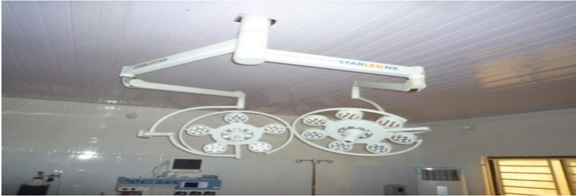
Picture 35: Procured LED Operation/Surgery Light at FMC, Yola
