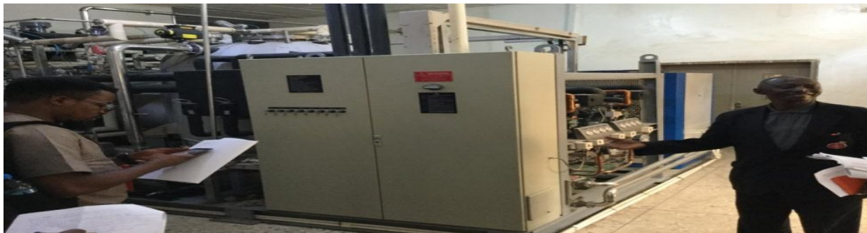
Picture 3: Refurbished Freeze Dryer Machine at NVRI, Vom
