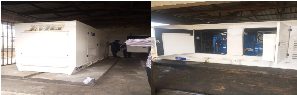
Picture 34: Procured Generating Sets at Federal Medical Centre (FMC) Yenegoa
