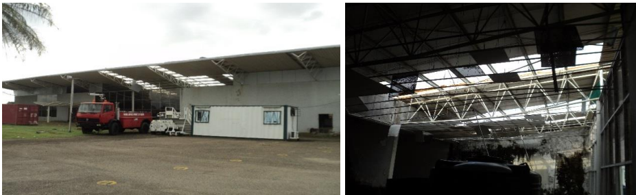
Picture 45: The deteriorated terminal building at Makurdi Airport
