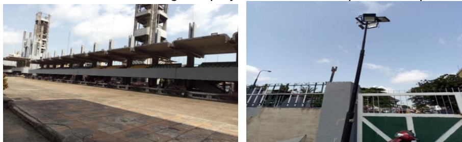
Picture 51: Installed Lighting and Fittings at the Parade Ground in TBS, Lagos
