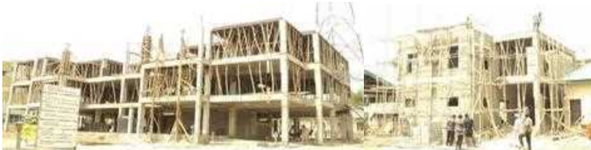
Picture 77: Ongoing Construction of Administration Building Phase II and Store Outlet at the ARCN HQTRS, Abuja.
