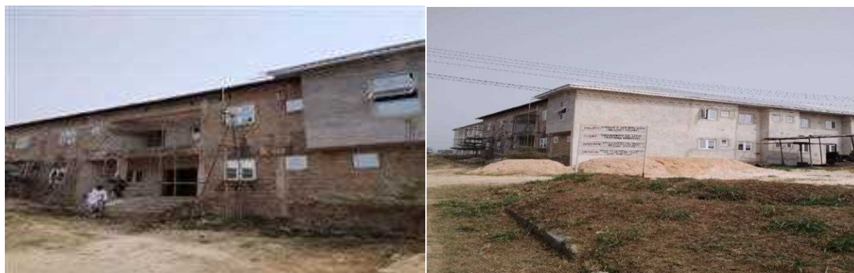
Picture 71: Ongoing expansion of antenatal Block at University of Uyo, Teaching Hospital, Akwa Ibom State.
