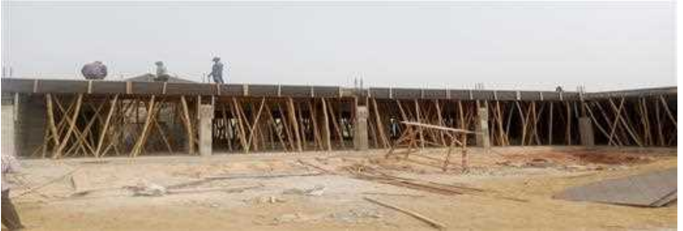
Picture 44: Ongoing Construction of Academic Building for the Faculty of Environmental Sciences at Alex Ekweme Federal University Ndufu Alike, Ebonyi.
