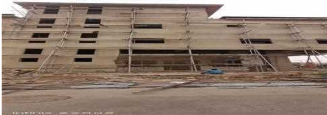
Picture 62: Ongoing Reconstruction of Ophthalmic Complex at the Federal Medical Centre (FMC), Jabi.
