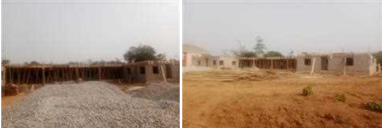
Picture 45: Ongoing Construction of One-Storey Staff Office Accommodation at Alex Ekwememe Federal University Ndufu Alike, Ebonyi.
