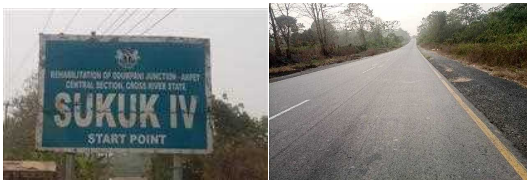
Picture 13: Ongoing: Rehabilitation of Calabar-Ugep-Katsina Ala Road, Section II in Cross River State.
