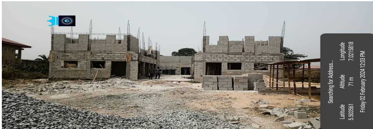
Picture 69: Ongoing construction of the hospital central storage facility at FMC, Owerri.
