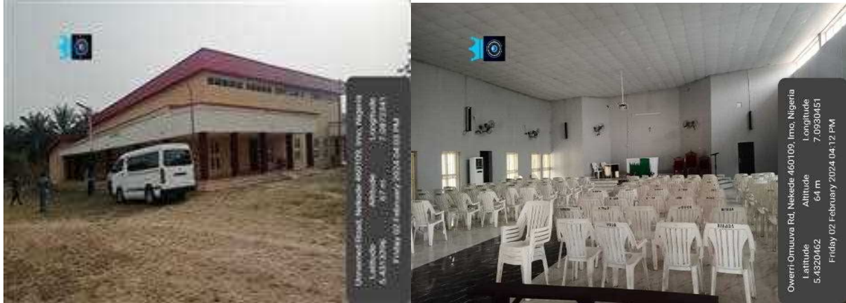
Picture 28: Ongoing rehabilitation of Anambra Imo River basin development authority’s multi-purpose hall and training Centre.
