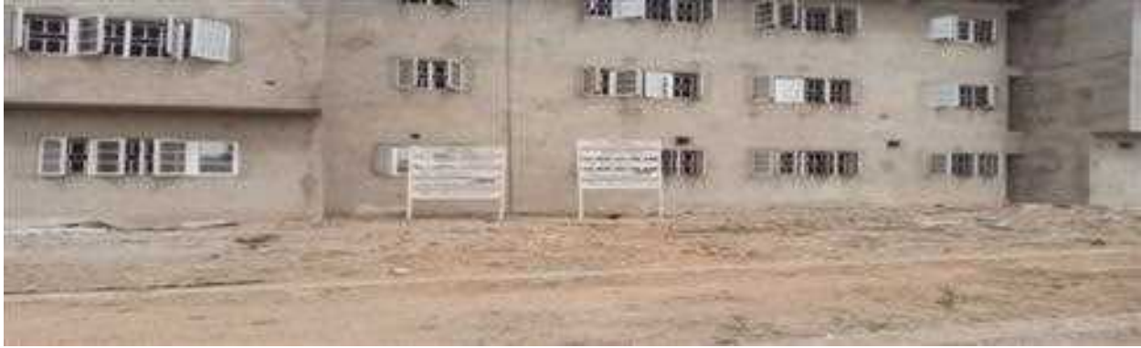
Picture 32: Ongoing Construction of Physiology Laboratory Medical College at Modibo Adamawa University.
