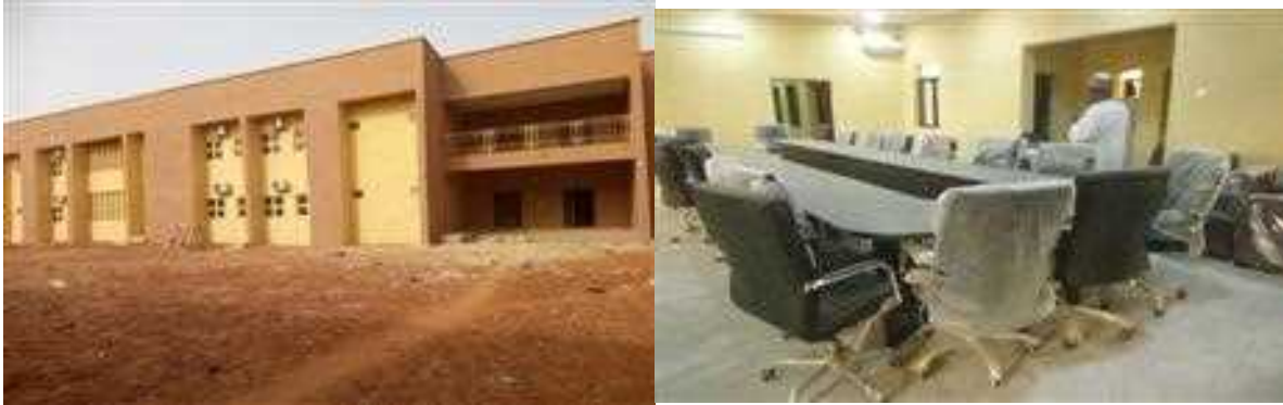
Picture 33: Ongoing construction of faculty of Veterinary Medicine at Usman Danfodio University, Sokoto.
