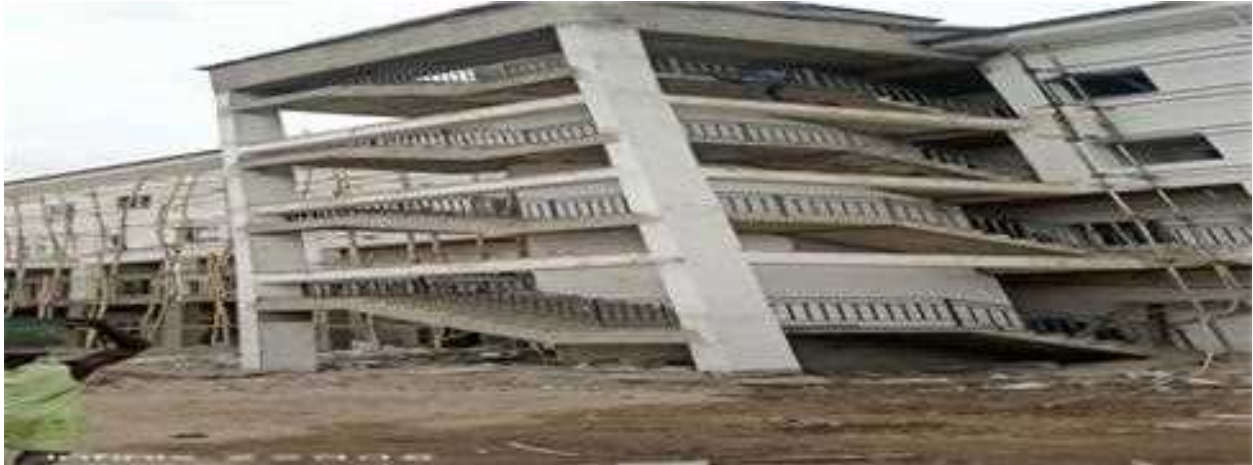
Picture 61: ongoing construction of Clinical Services Block at the Federal Medical Centre, Abuja
