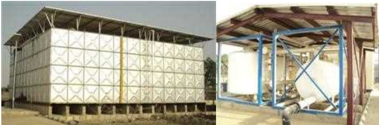
Picture 18: Constructed Water Supply Project at the Gashua Town, Yobe State.
