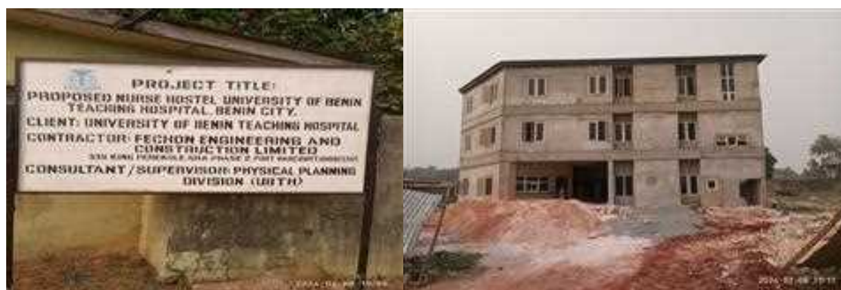
Pictures 74: Ongoing construction of Student's Hostel Complex at University of Benin Teaching Hospital
