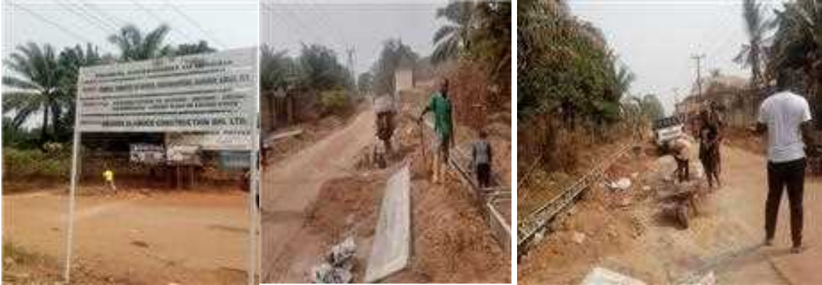
Picture 14: Ongoing Rehabilitation of Akpugo – Ndiuno – Amugo – Ihunekuagu – Obuno Road in Nkanu West LGA in Enugu State.
