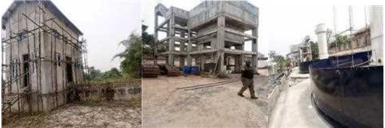
Picture 26: Completion of construction of Ota water supply project in Ogun state
