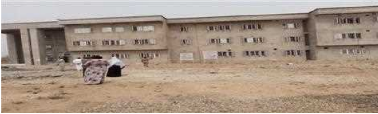
Picture 31: Ongoing Construction of pharmacology laboratory, medical college at Modibo Adamawa University.
