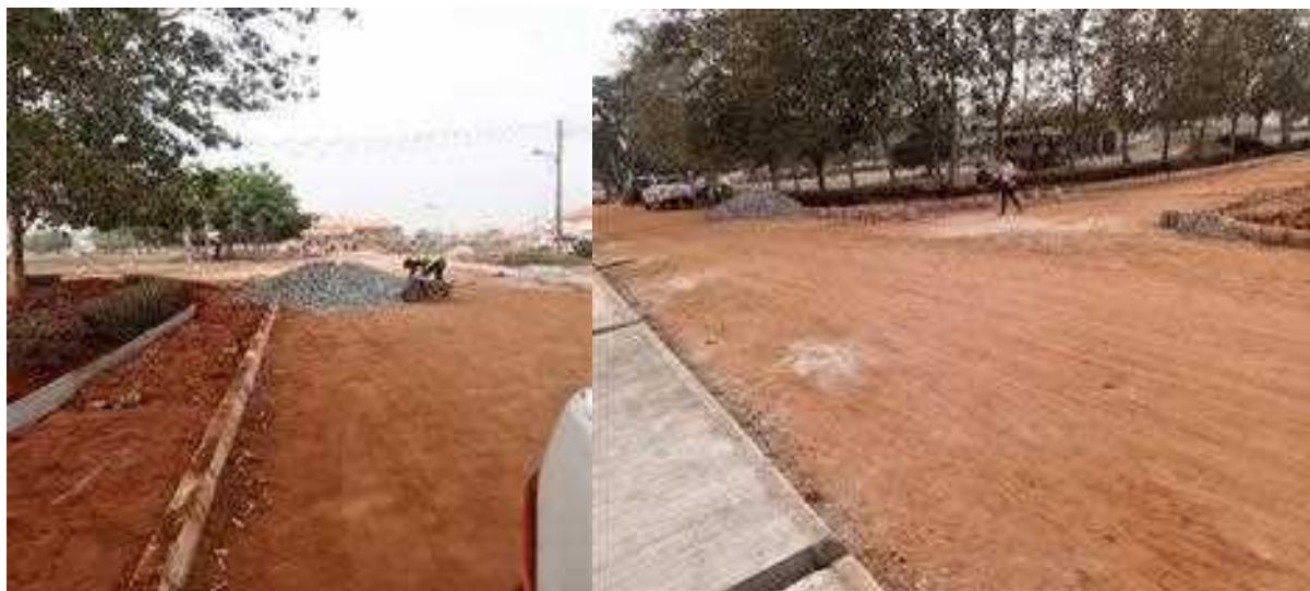
Picture 40: Rehabilitation of 600 metres Road from UBA junction to Edo-mass communication linking multipurpose hall road.
