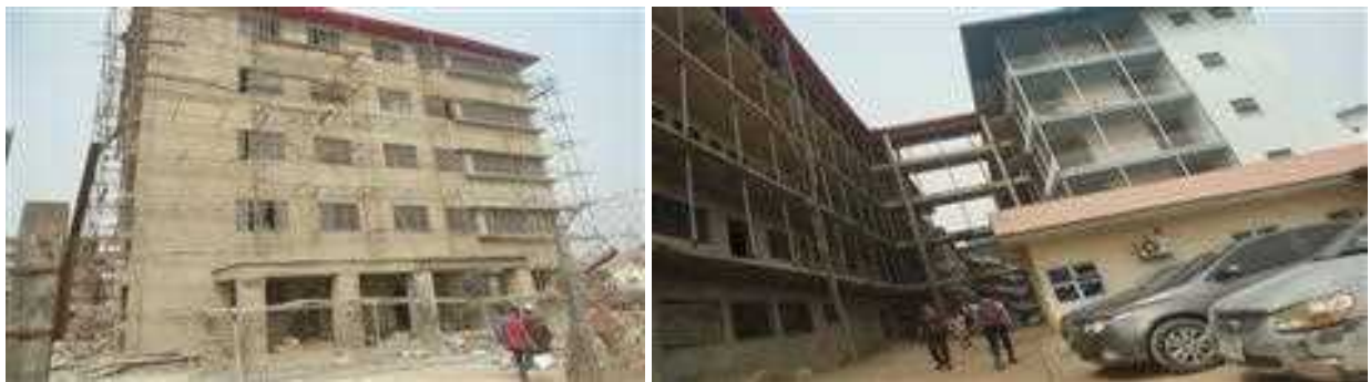
Picture 66; Ongoing extension / equipping of emergency clinic (Phase I) at University College Hospital, Ibadan.
