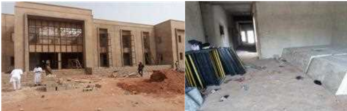
Picture 55: Ongoing Construction and Furnishing of NHIS/GOPD Complex at Federal Teaching Hospital, Gombe.
