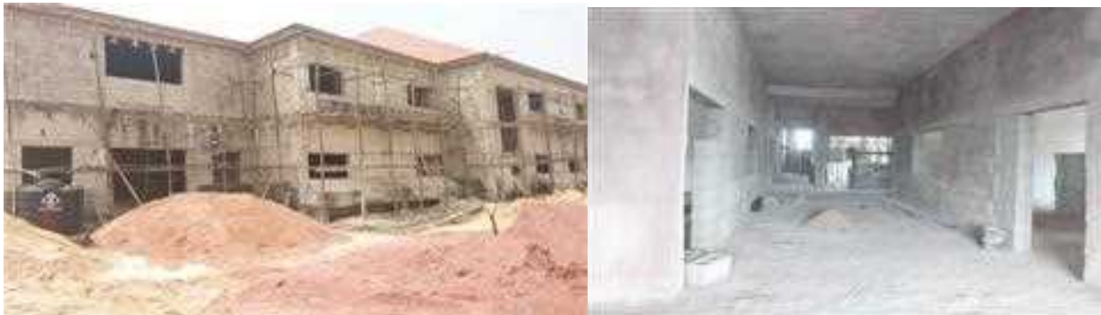
Picture 43: Ongoing completion of Centre for energy and power system research building at Federal University of Technology Owerri.
