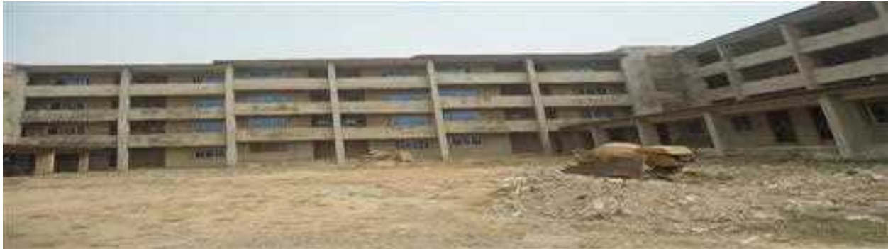
Picture 67: Ongoing Completion of House Officers Residence III (Phase 1) at University College Hospital, Ibadan.
