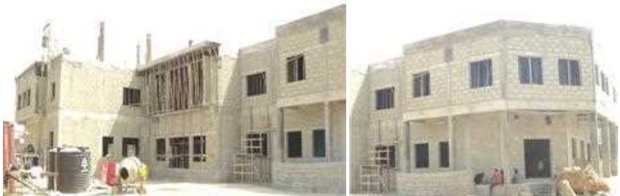
Picture 47: Ongoing construction of ICT Centre at University of Maiduguri Teaching Hospital.
