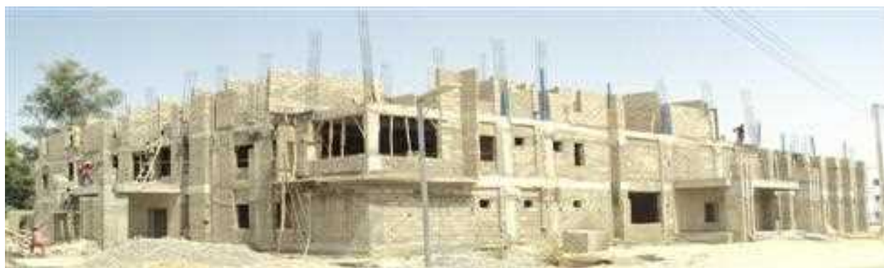
Picture 48: Ongoing construction of New Cardiac Centre at University of Maiduguri Teaching Hospital (UMTH), Maiduguri.
