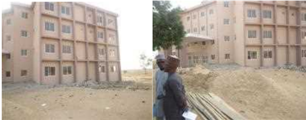
Picture 35: Ongoing construction of Senate Building at Federal University, Gusua, Zamfara State.
