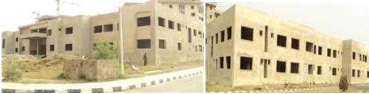
Picture 1: Ongoing construction of the medical centre at NDC permanent site, Piwoyi, Phase II.
