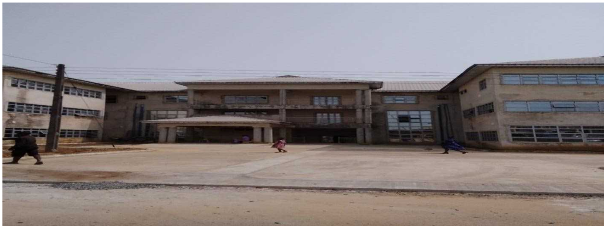
Picture 70: Ongoing completion of Laboratory building at University of Uyo Teaching Hospital, Akwa Ibom State.
