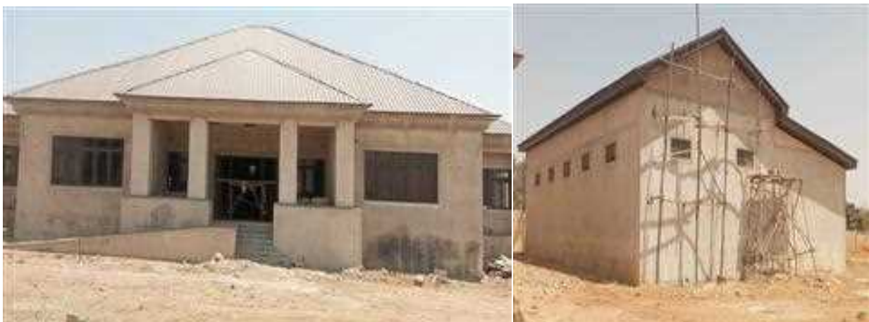
Picture 52: Ongoing construction of administrative building and store at the NAFDAC zonal office in Jos – Plateau State.
