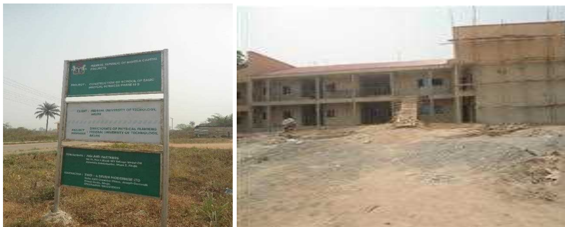
Picture 41: Ongoing Construction of school of Basic Medical Sciences Building (Phase IIIB) at Federal University of Technology, Akure.
