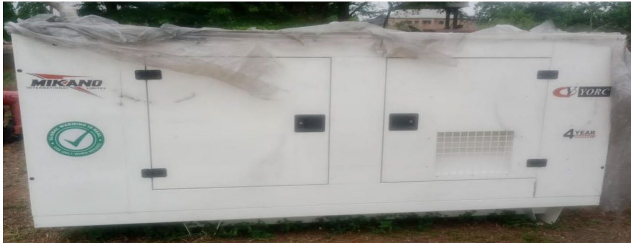
Picture 195: Procured 50KVA generator set at Federal College of Education (Technical), Umuze, Anambra State.
