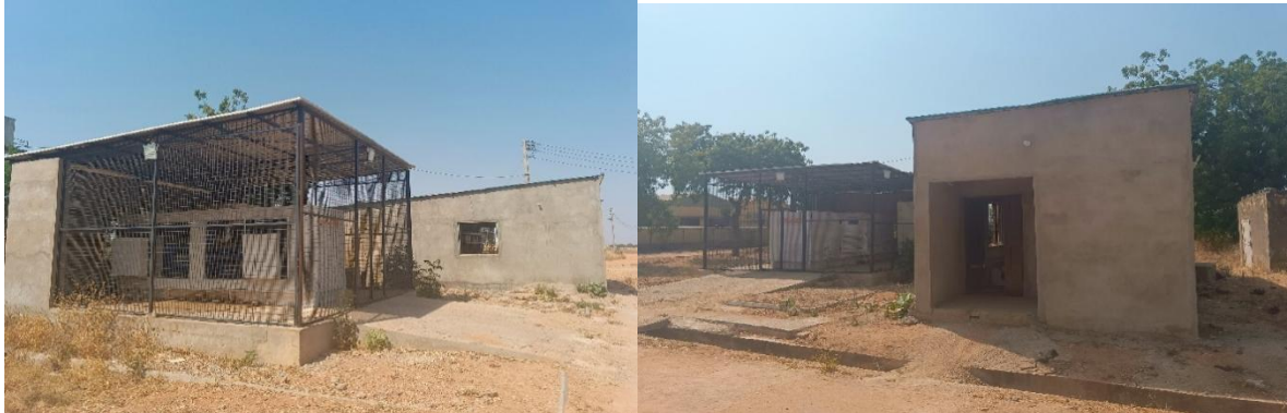
Picture 53: Emergency Renovation of Power House, Generator Base, Procurement and Installation of 500KVA Generator at Federal Teaching Hospital, Katsina.
