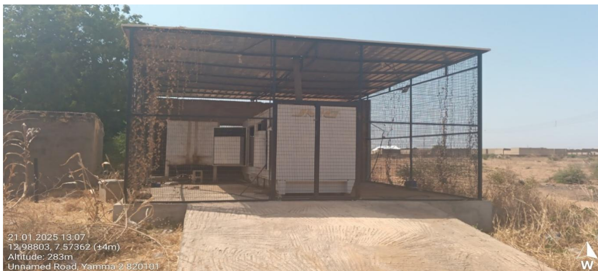
Picture 54: The Purchased 500KVA Backup Generator at Federal Teaching Hospital, Katsina.
