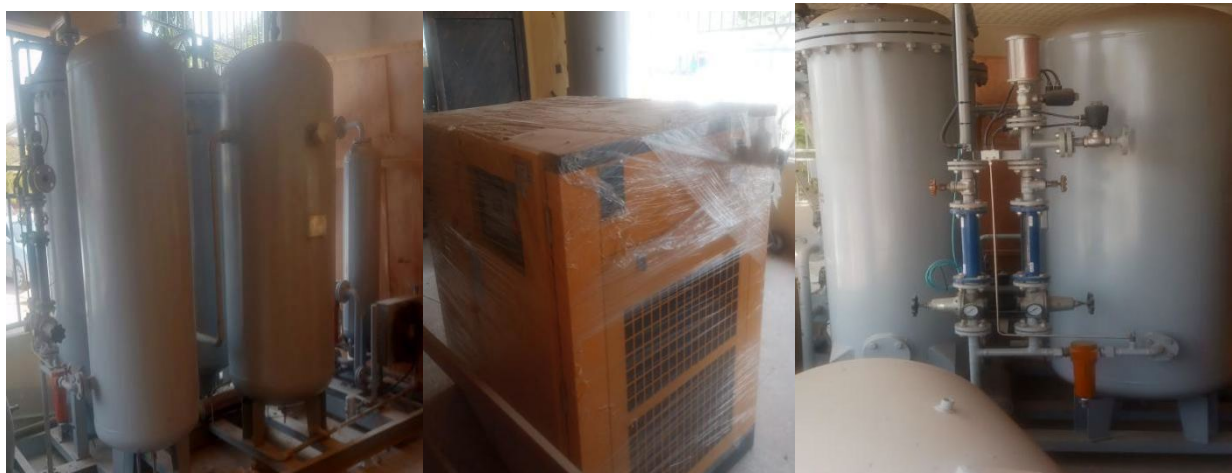
Picture 65: Procured Air Compressor Refrigerated Dryer, Activated Carbon Filter/Oxygen Buffer Tank and Pressure Swing Absorption (PSA ) at National Fistula Hospital, Abakaliki.
