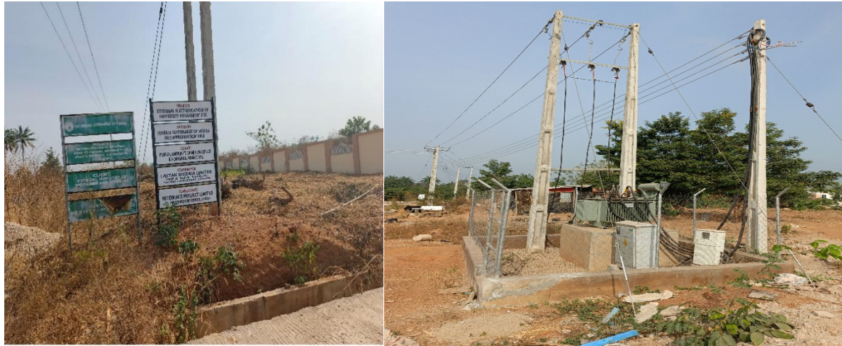
Picture 149: Procured and Installed Transformer at Federal University of Health Sciences, Ila-Orangun.
