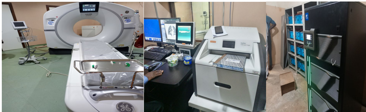
Picture 46: Rehabilitated/renovated CT room, and installed 64 slices CT scan machine with accessories
