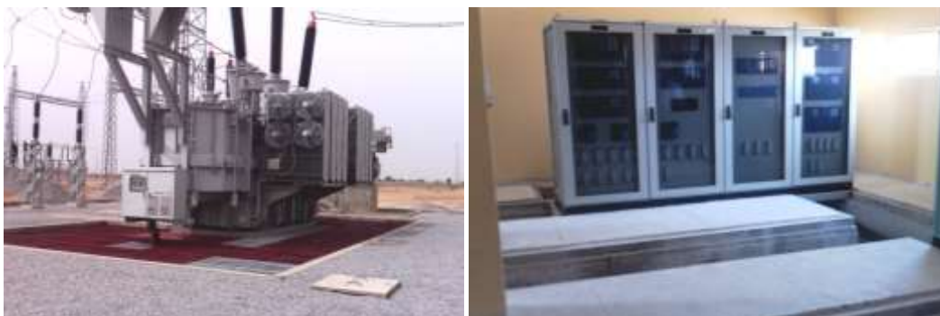
Picture 9: Maiduguri 330/132KV substation power transformer and associated switch gear.
