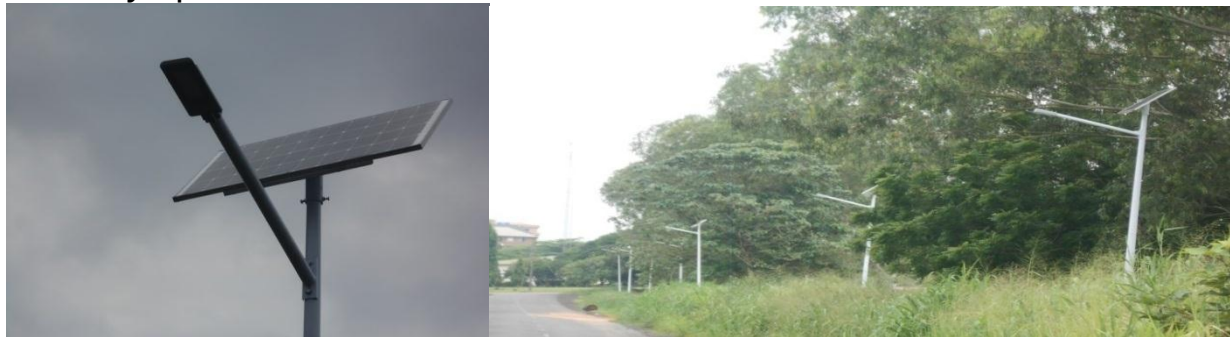
Picture 18: Part of the Solar Energy System installed at Metallurgical Training Institute, Onitsha
