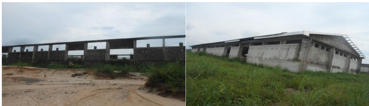
Picture1: Transit Shed, Warehouse and Workshop Structures Stalled at the River Port Site, Oguta
