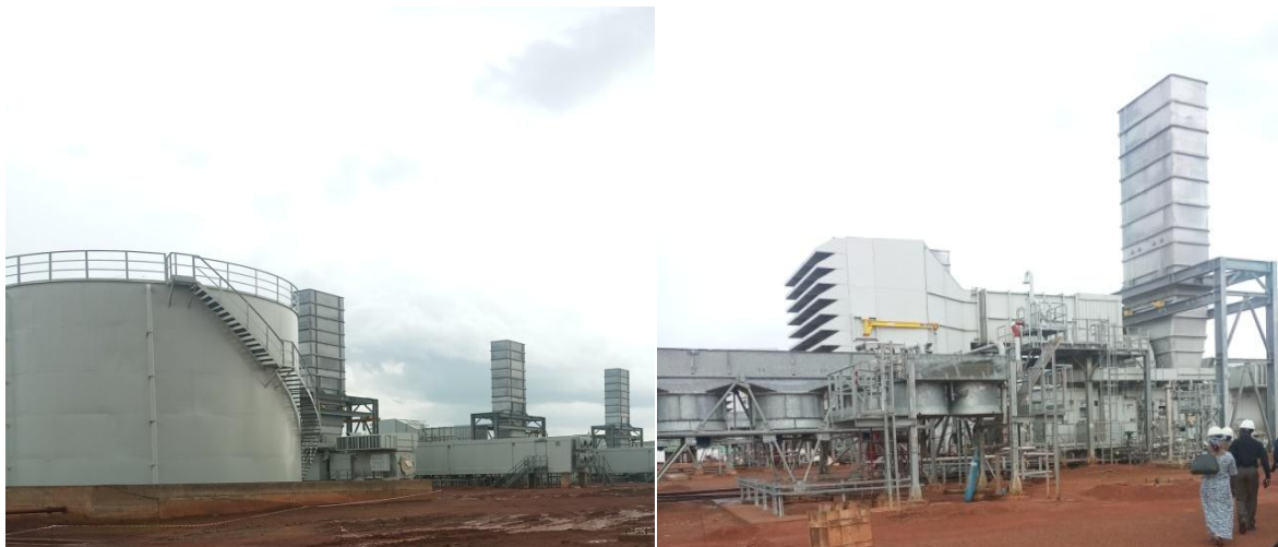
Picture 15: Plant Components at 215 MV Dual Fired LPFO/ Gas Power Plant, Kaduna
