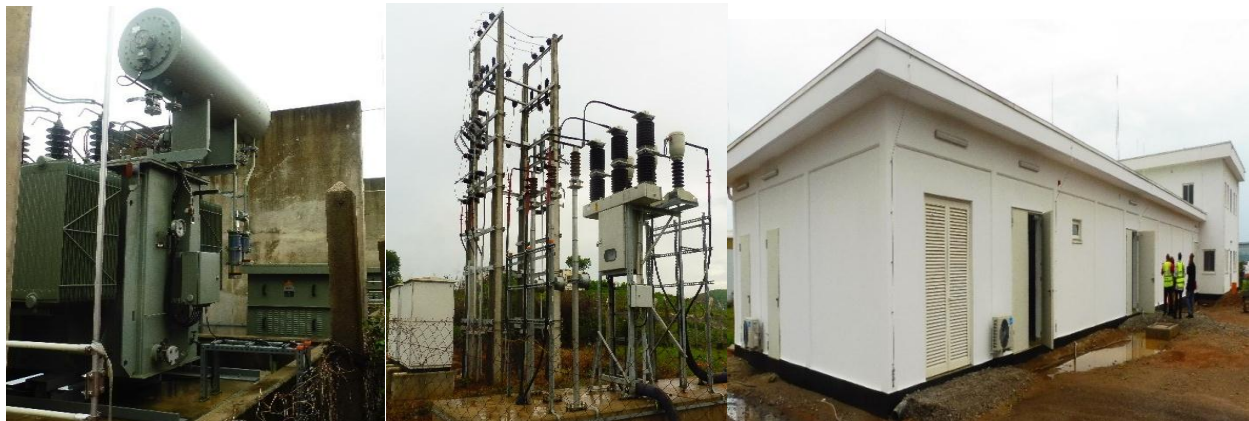
Picture 17: Newly Installed 7.5 Mega Volt Amps (MVA) Transformer and Powerhouse with an adjoining Administrative Building at NAIA Abuja
