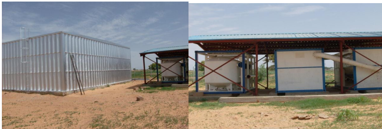
Picture 19: Installed Water Tank and Water Treatment Plant at Shagari Dam Area, Sokoto
