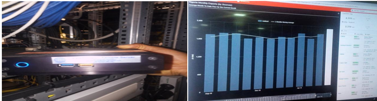
Picture 53: Procured Remote Transmission Units (RTU) at DPR Headquarters, Lagos
