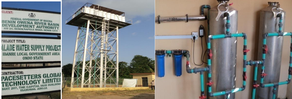
Picture 18: Completed Overhead Tank and Control Room at Idanre Water Supply Scheme
