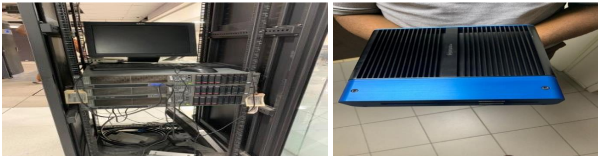
Picture 61: Procured Remote Transmission Units (RTU) at DPR Headquarters, Lagos.
