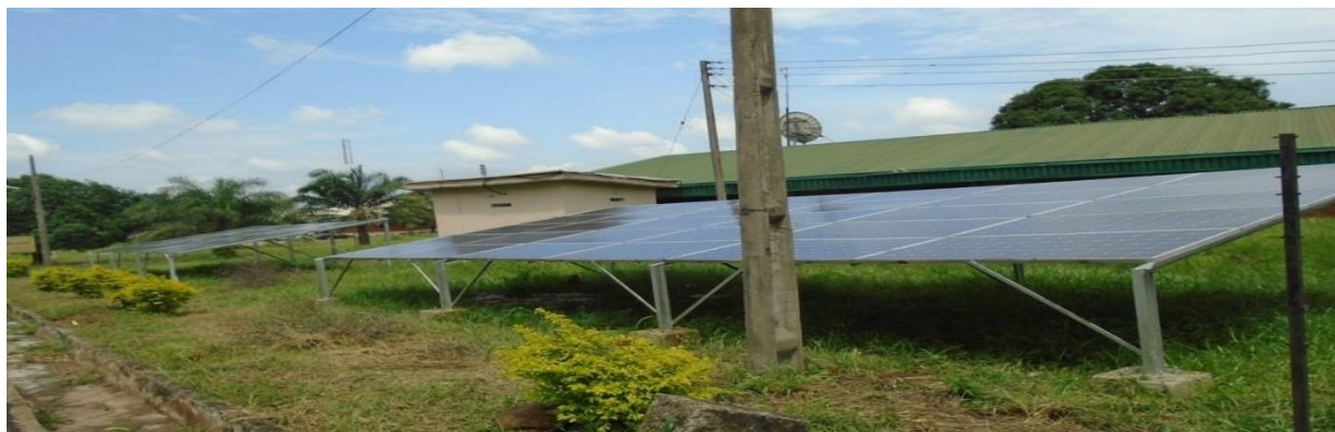
Picture 64: Installed Solar Energy Panel at Metallurgical Training Institute, Onitsha
