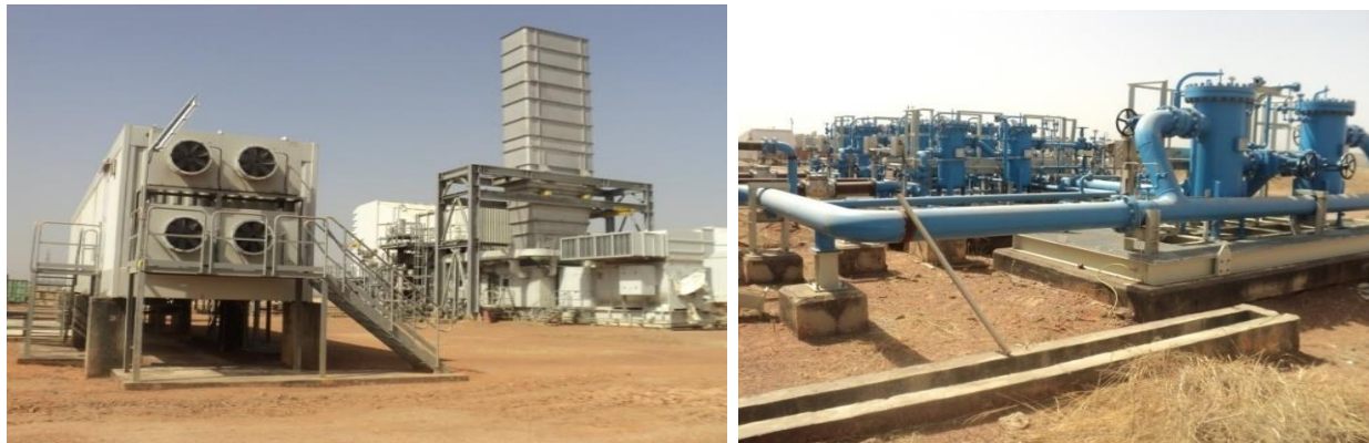
Picture 6: One of the Gas turbines, Switch Yard and Filtration Components Installed at the Project site, Kaduna
