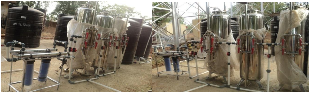
Picture 22: The Installation of Water Treatment Plants almost completed at the River Basin Headquarters' Complex, Sokoto
