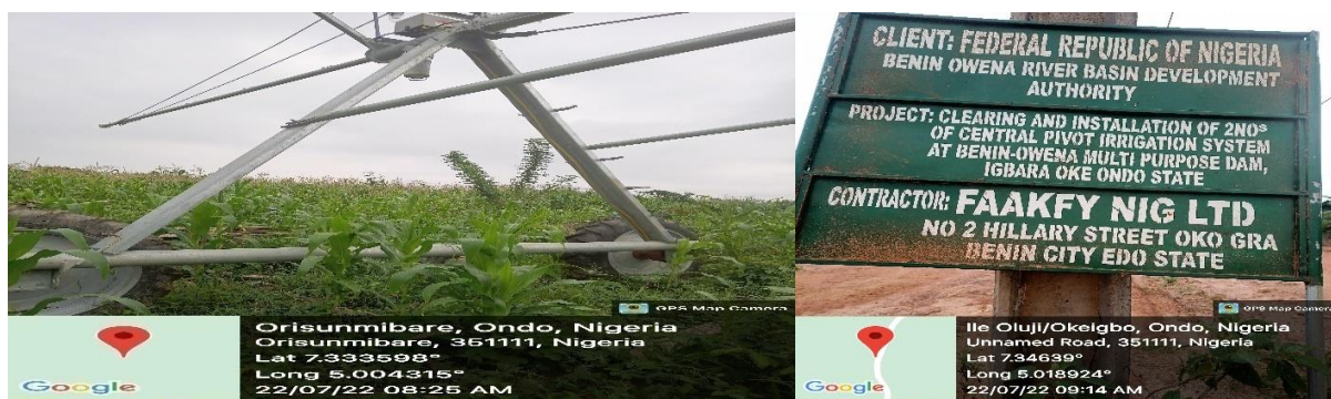
Picture 17: One of the Procured CPIS at the Owena Multipurpose Dam, Akure
