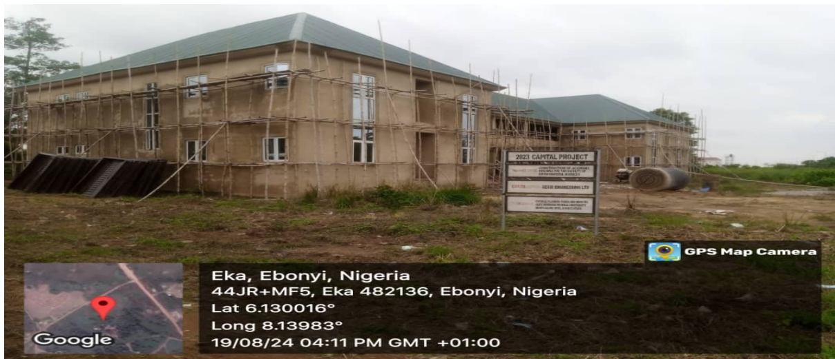
Pictures 50: Ongoing Construction of Academic Building for the Faculty of Environmental Sciences at Alex-Ekwueme Federal University Ndufu Alike, Eboyi State.
