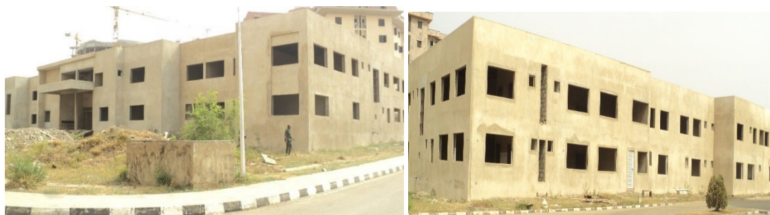
Picture 65: Ongoing construction of the medical centre at NDC permanent site, Piwoyi, Phase II at National Defence College, Abuja.
