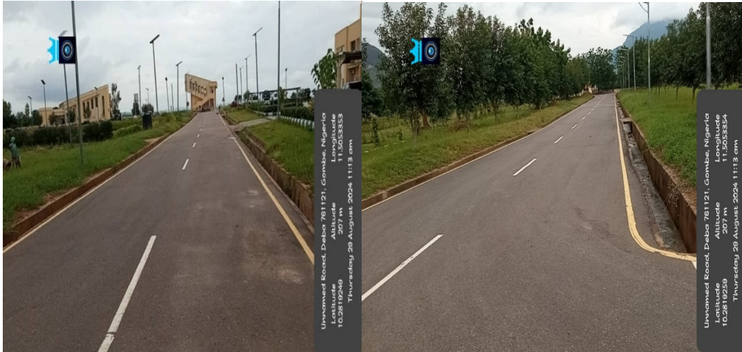
Picture 70: Rehabilitation of internal roads at the Federal College of Horticulture, Dadin-Kowa.
