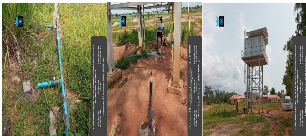
Picture 52: Constructed borehole, solar water tank and installation of irrigation pipes at Upper Benue River Basin Development Authority.
