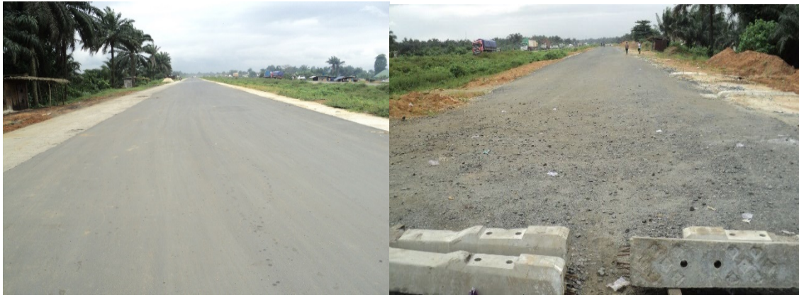
Picture 58: Ongoing Rehabilitation of Enugu- Port-Harcourt Dual Carriageway, Section IV: (Aba-Port Harcourt) in Rivers State.
