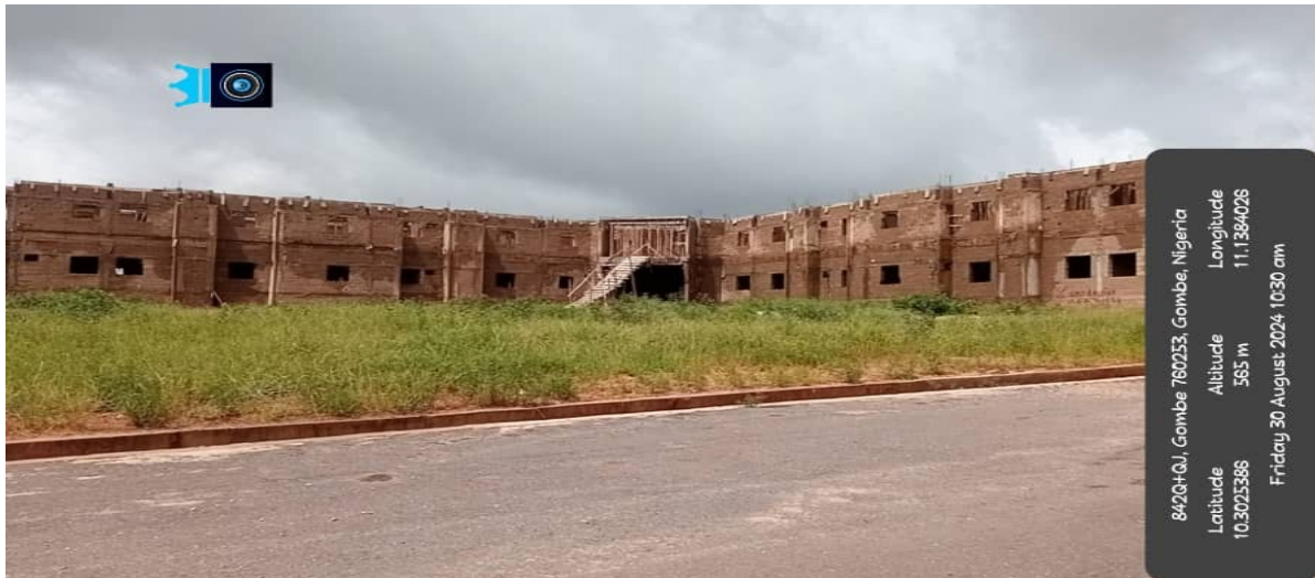
Picture 7: Ongoing Construction of Laboratory Complex Phase 1 at Federal Teaching Hospital Gombe.
