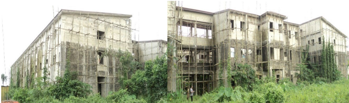
Pictures 25: Ongoing completion of Interns Hostel at University of Port Harcourt Teaching Hospital (UPTH), Rivers State.
