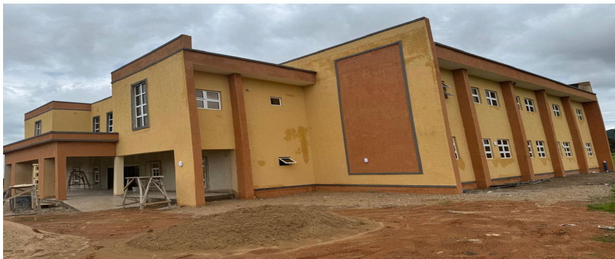
Picture 30: Ongoing Construction of Offices and furnishing of offices, lecture halls, and laboratories for the faculty of Natural Sciences at University of Jos.
