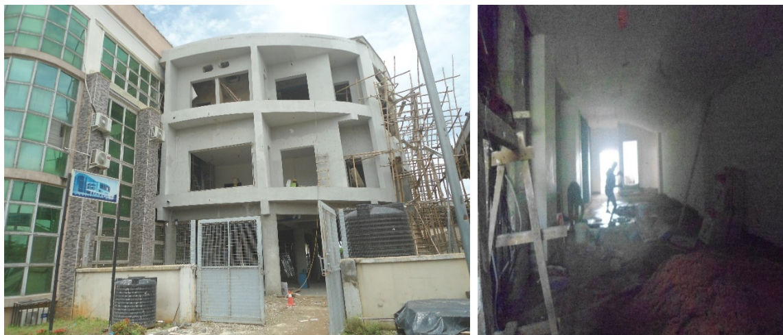
Picture 51: Ongoing Construction of Senate building at National Open University of Nigeria, Abuja.
