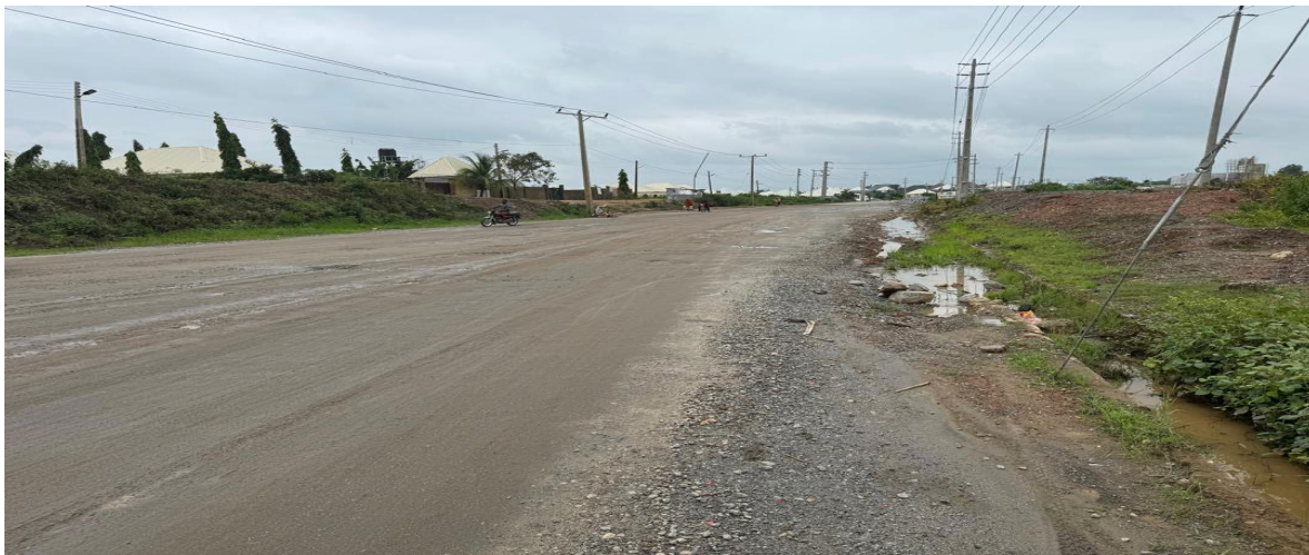
Picture 55: Ongoing Rehabilitation of Keffi – Nasarawa – Toto Road in Nasarawa State, Contract No. 7485.
