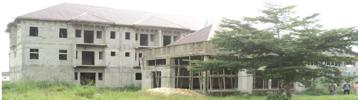
Picture 24: Ongoing Construction and Equipping of Physiotherapy Department at the University of Port Harcourt Teaching Hospital (UPTH).
