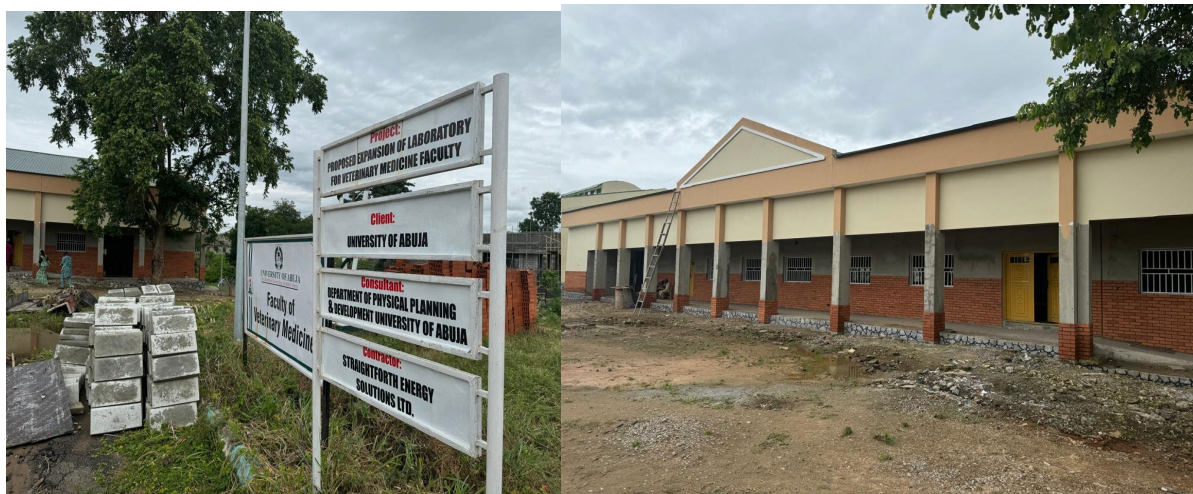
Picture 28: Completed expansion of Faculty of Veterinary Medicine Laboratory at University of Abuja.
