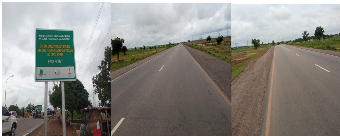
Picture 57: Ongoing Rehabilitation of Cham-Numan section of Gombe - Yola Road in Adamawa State.
