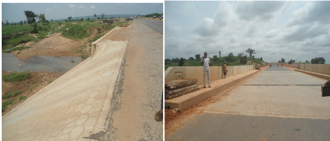
Picture 59: Ongoing retaining wall /concrete stone pitching at dualization of Ilorin-Jebba-Mokwa/Bokani in Niger state.
