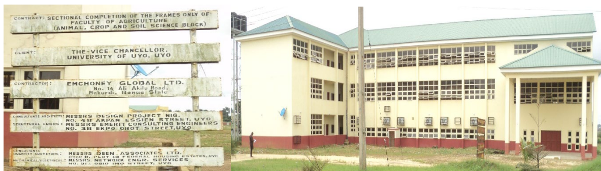
Picture 42: Ongoing Completion of Faculty of Agriculture Laboratory Block (Phase I) at University of Uyo, Akwa Ibom State.
