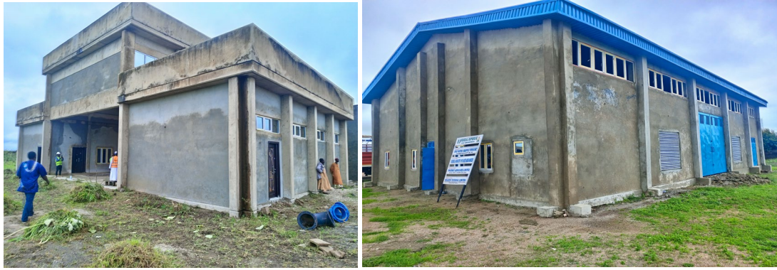
Picture 54: Ongoing construction of the workshop building and Buster station at Biu water supply.
