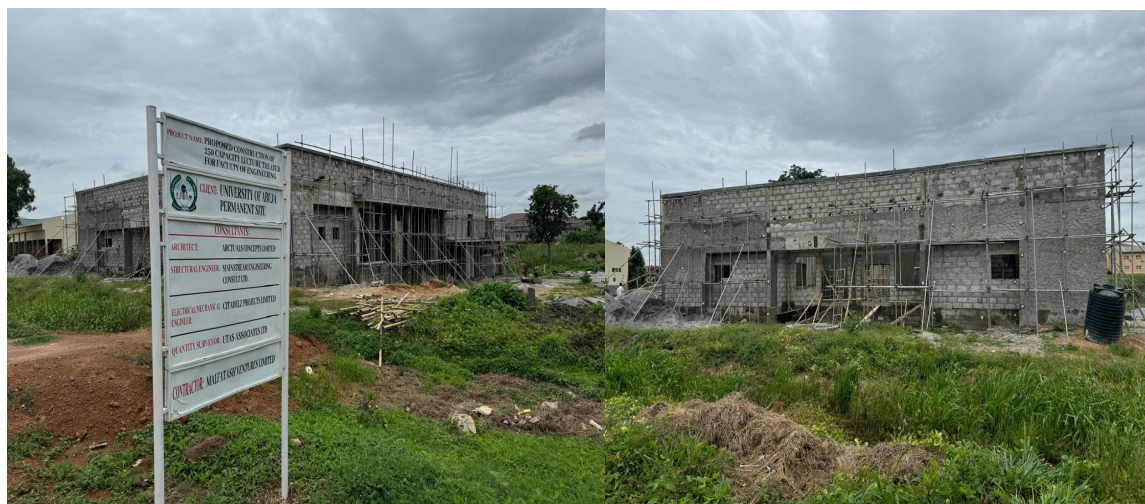
Picture 29: Ongoing Construction of 250 Capacity Lecture Theatre for Faculty of Engineering at University of Abuja.
