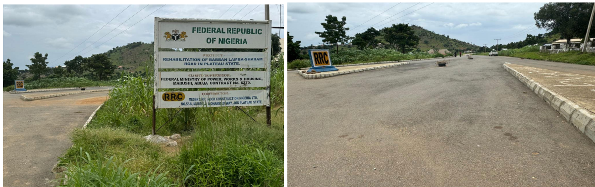
Picture 56: Ongoing Rehabilitation of Babban Lamba – Sharram Road in Plateau State Contract No. 6270.
